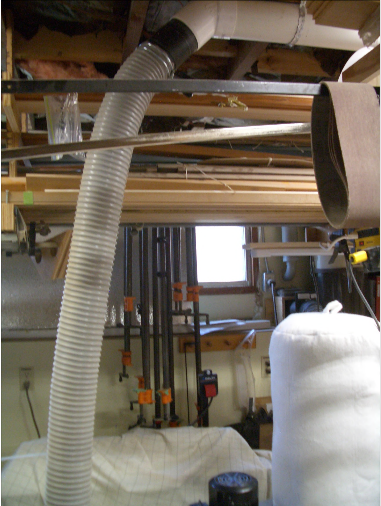
Figure 2 This shows the connection from the dust collector's hose to one end of the pipe and fittings in the ceiling.
