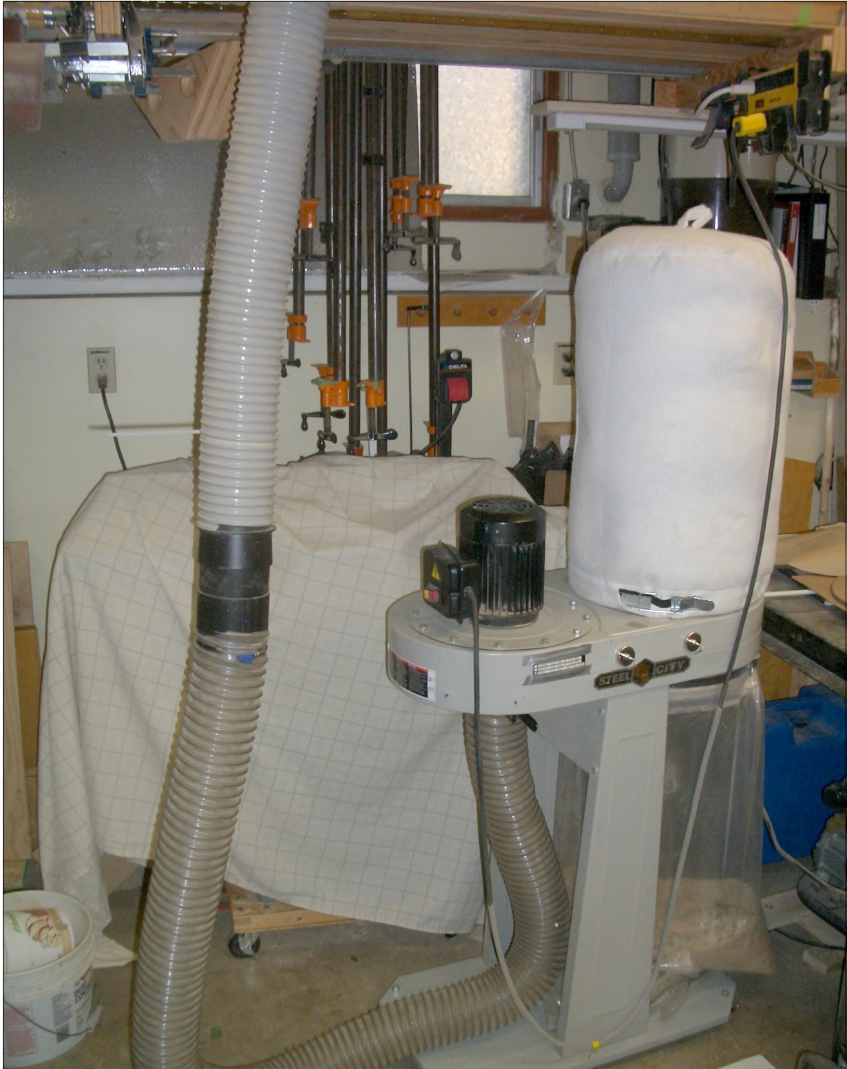
Figure 1 This shows how my dust collector's vacuum is directed up to the PVC pipe in the ceiling.
