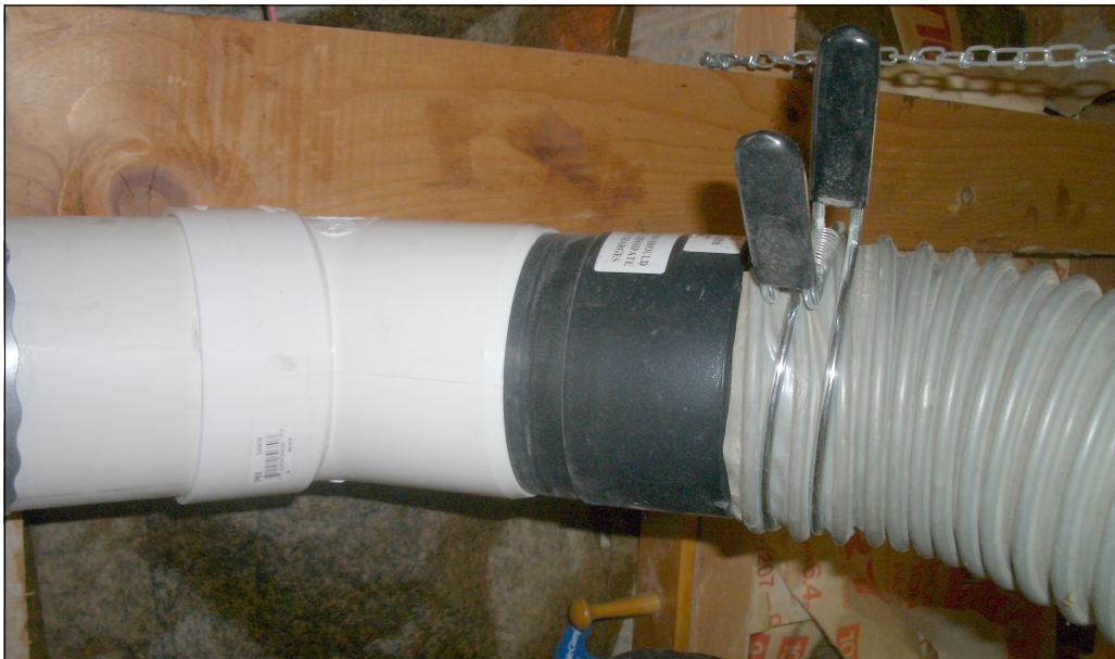
Figure 4 This is a closer view of the main transitions at each end. From left to right, the pipe has the female end of the sewer elbow over it then the splice (turned down in diameter) slipped inside the male end of the sewer elbow. Finally, the hose is installed on the splice and held in place by the squeeze hose clamp.
